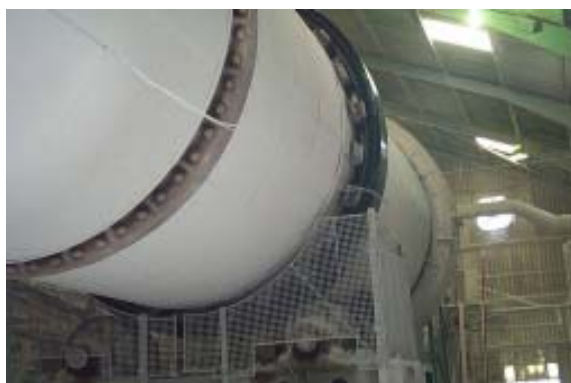
Metallock Engineering in-situ machined two 4-metre diameter, 300mm wide china clay drying kiln tyres for Imerys Minerals to eliminate vibration caused by severe tyre wear.
