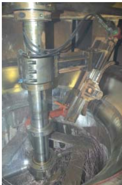
Metallock successfully machined a complex runner chamber profile at Culligran hydro power station for Weir Engineering Services.
